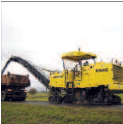
Quick, accurate incutting on secondary road pavement repairs helped by marks on the side plates.
