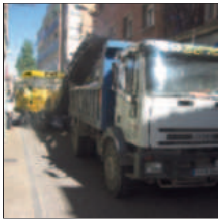
Even in tight spots: an excellent view to the milling edge and over the construction site.
